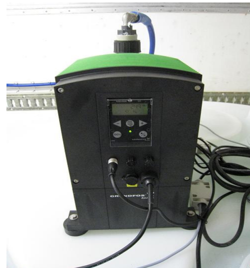
The dosing pump
